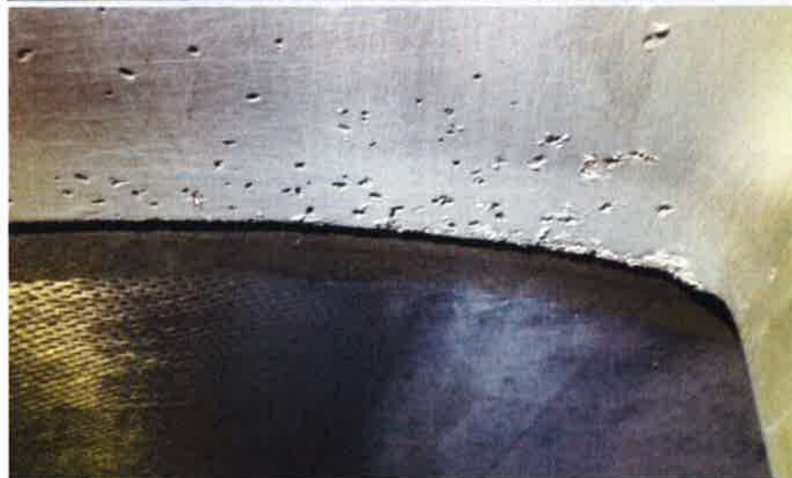
Figure 3 – Photographs to show the reported corrosion
