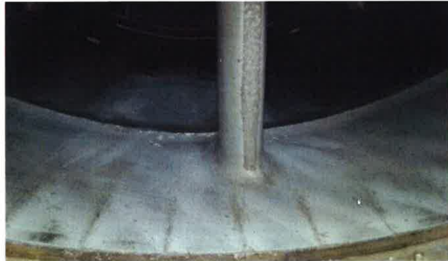
Figure 2 – Photographs to show the reported corrosion
